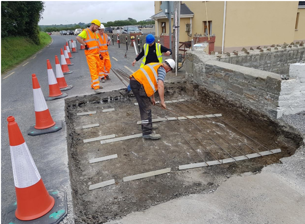
Figure 29 Typical Installation of a Reinforced Concrete Slab over a Stone Clapper Structure
